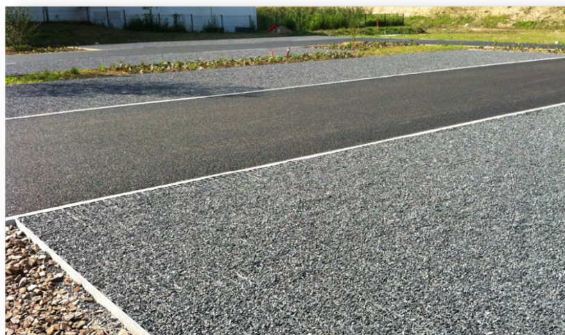
Source : INFRA Services
